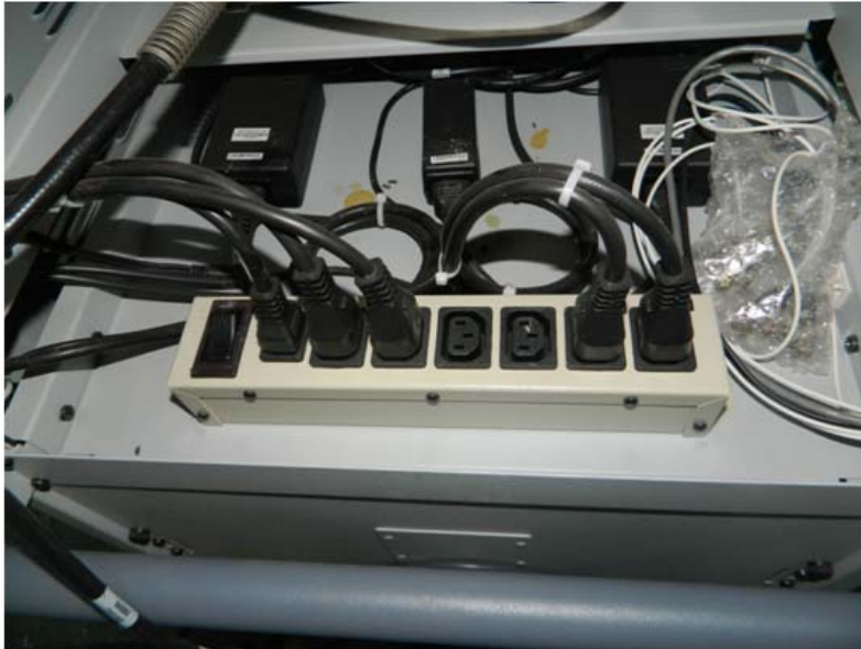
Fig. 7: Power strip on the vision cart
